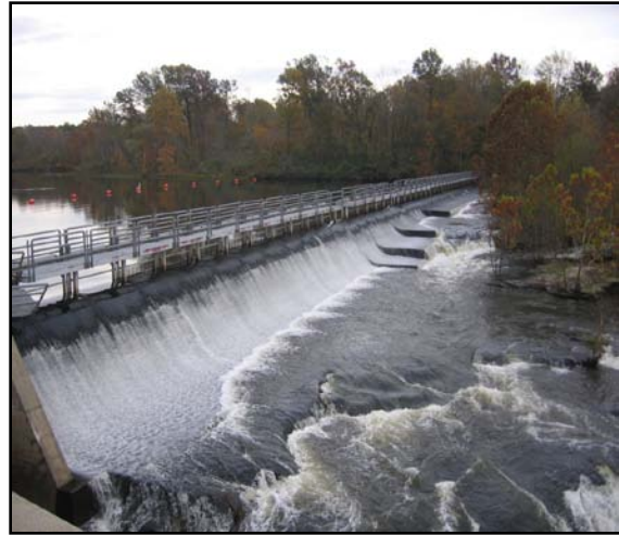
This dam at Crab Orchard NWR in Illinois requires additional dam safety repairs.
