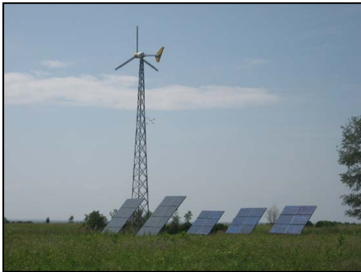
Pictured above is a wind turbine and solar array at Eastern Neck National Wildlife Refuge in Maryland, which provides the renewable energy necessary for one of the refuge office buildings to approximate zero net energy use. Pictured below is an electric vehicle in use at Chincoteague National Wildlife Refuge.
